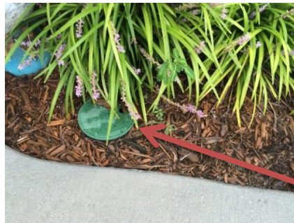
Shut off valve inside
