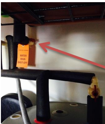
Shut off valve
